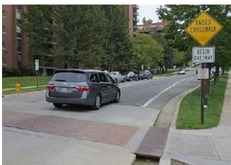
Raised crosswalk with chase cover Source: FHWA via Jeff Gulden
